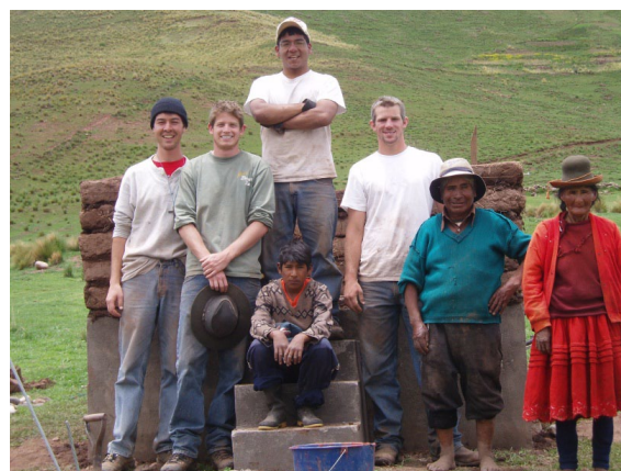
Adam Ureneck '04 in the Puno region of Peru helping to install eco-toilets
